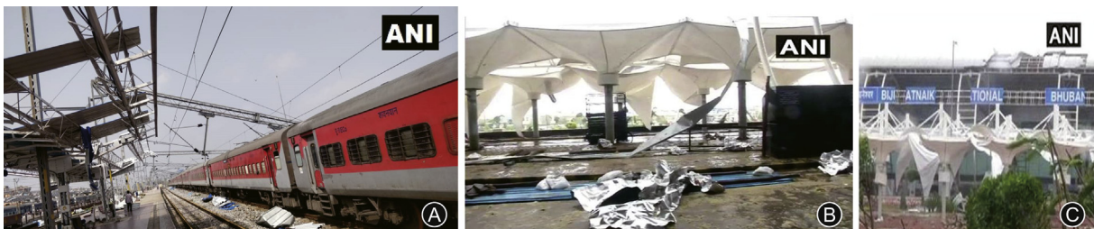
Fig. 6. Massive damage to the railway station and airport. Source of figures: Agency France Press and Asian News International.
