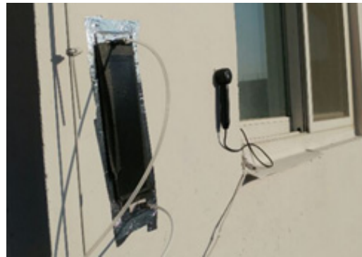
Figure 9. Installed photoreactor and UV radiometer on the rooftop.
