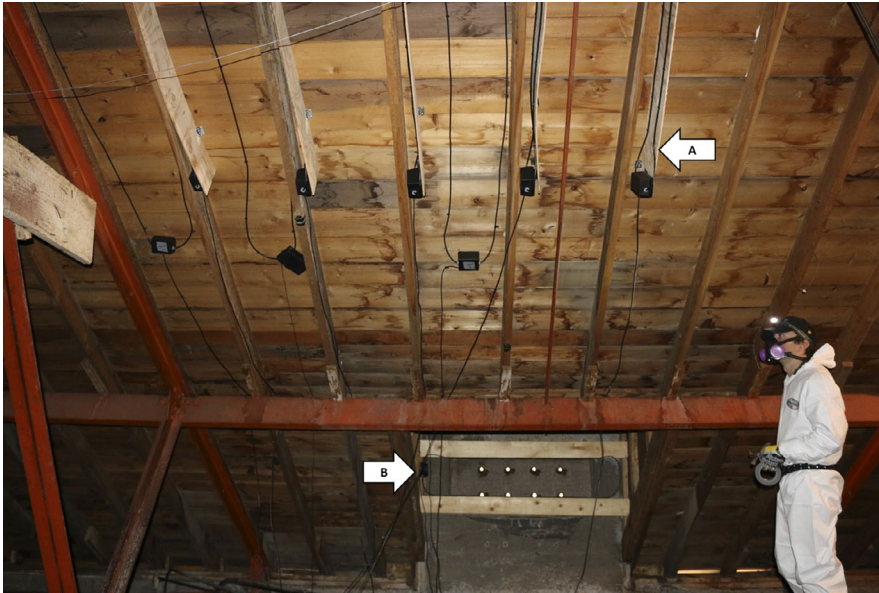
FIGURE 2 PIT tag antennas placed along an attic ceiling (arrow “A”) and entryway antennas that bats traverse through to access the roost (arrow “B”), inside a little brown myotis maternity roost in Yellowstone National Park, USA. Ceiling antennas were placed at two different orientations. Antennas were positioned perpendicular to the attic ceiling on plywood segments and flush to the attic ceiling to increase tag readability through different orientations of antennas relative to PIT-tagged bats. Read ranges of antennas did not overlap
