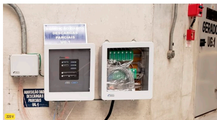
Figure 5. Installation panel for this system at the plant.
