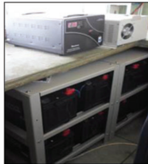
Inverter and Batteries
