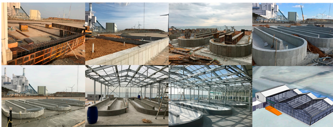
Figure 12. Images showing the construction of the semi-open raceway system (ORS) at the selected site in Incheon, Korea.
