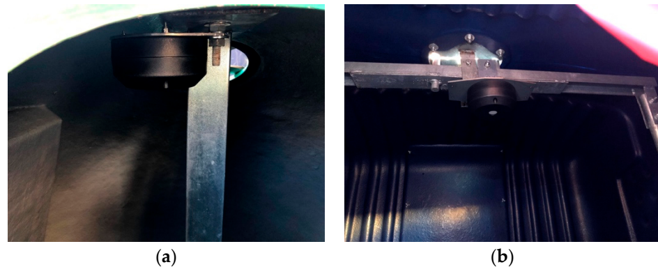
Figure 7. Dingtek DF702 installed in the containers: (a) installed in an Iglô; (b) installed in the Cyclea.
