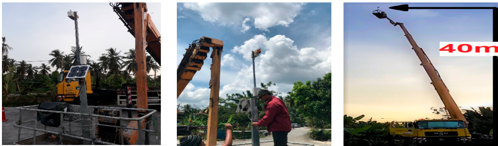
Figure 6. Completed transmission node enclosed in a weatherproof box and fixed on top of a Skylift crane at a height of 40 m.
