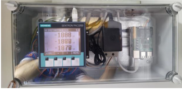
Fig. 9. Power monitoring and Raspberry PI hardware.
