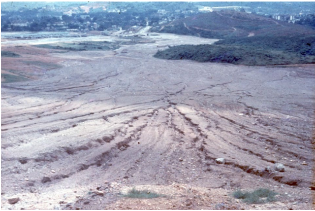
Fig. 11 View from the Damansara Heights construction site towards the centre of Kuala Lumpur (top left) in 1969 showing rapidly developing erosion gullies that led to blocked channels and flooding downstream every time heavy rain occurred (photo by Ian Douglas)
