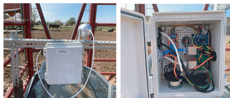
Figure 10. The junction electrical box implemented in each drinking station.
