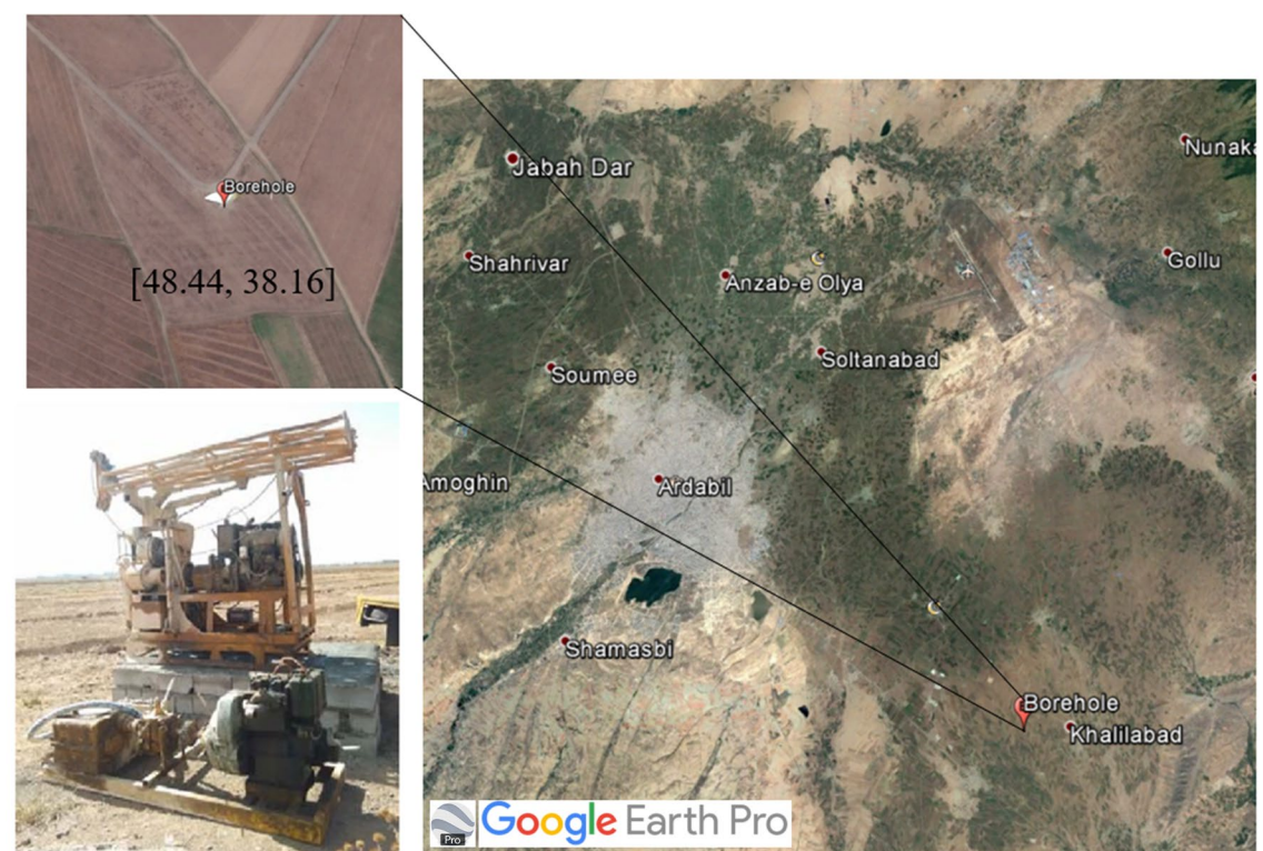
Figure 19. Drilling site of a borehole 105 m deep in the field. The map in this figure was created using the Google Earth/Pro version 7.3.4.8573 software ( https://earth.google.com/ ).
