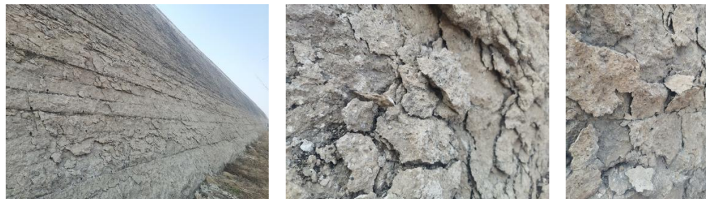
Figure 1. Diseases of the newly repaired earthen city walls.
