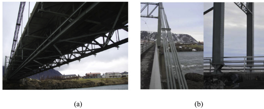
Figure 2. View of Olfusá suspension bridge (a) longitudinal & transverse trusses (b) cable arrangement [19, 20].
