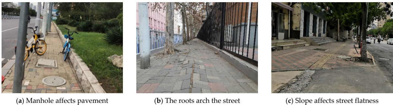
Figure 10. Reasons for uneven street surface.
