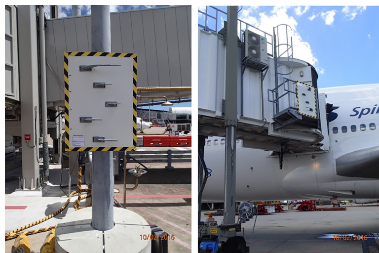
Fig 1. Pitot panels installed on gate light pole at domestic terminal (left) and on aerobridge at international terminal (right).
