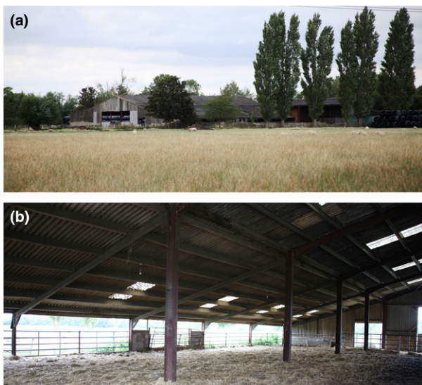
Fig. 2. External (a) and internal (b) view of cattle barn. Cattle barn utilised for habitat immunomarking. [Colour figure can be viewed at wileyonlinelibrary.com ]
