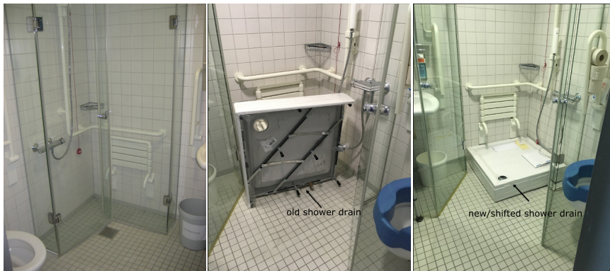
FIG 6 Removable and autoclavable shower insert to prevent direct contact with wastewater. Following unsuccessful eradication and new detections, removable shower tubs were installed to avoid backplash by shifting the shower drain away from the water jet from shower heads.
