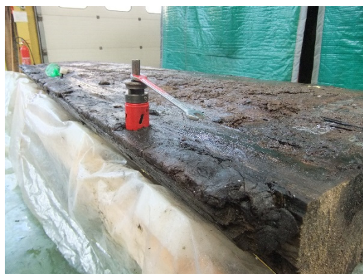
Figure 2. Sampling the core to evaluate the concentration of the acid precursors: coring drill around a nail position.
