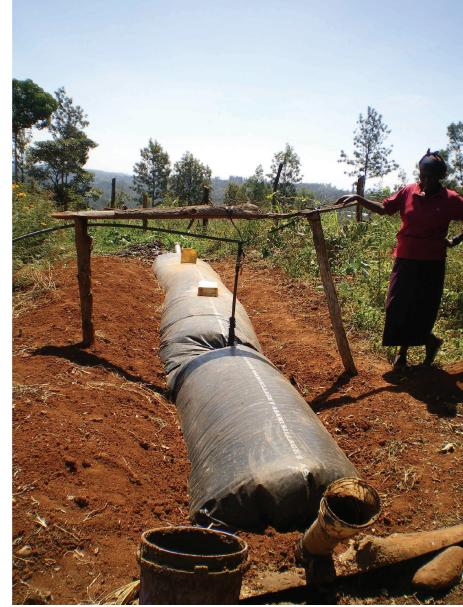
FIGURE 2: Biogas digester installed on a rural Kenyan smallholder dairy farm.
