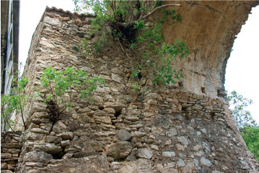
Figure 12 A bridge near Karytaina on the Peloponnese, Greece, northern springer of the third arch (from north to south) (photographer: Galina Fingarova).
