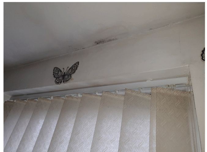
Fig. 2. An example of mould inside a living room.
