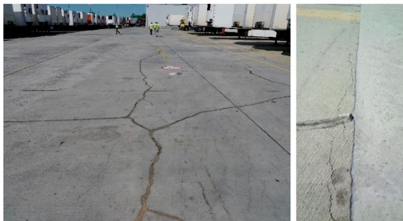
Figure 2. Damage examples: concrete pavement with cracks caused by shrinkage (left) and after repair with epoxy resin (right).
