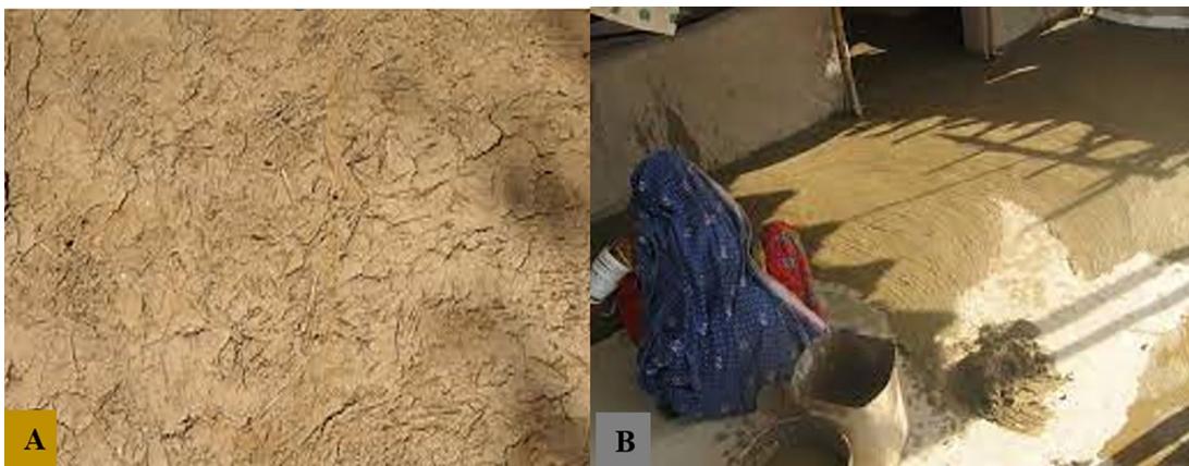
Figure 5. Cracked wall plastered with animal dungs (A) and a woman plastering floors using animal dungs with bare hands (B) in a rural setting of northwest Ethiopia.
