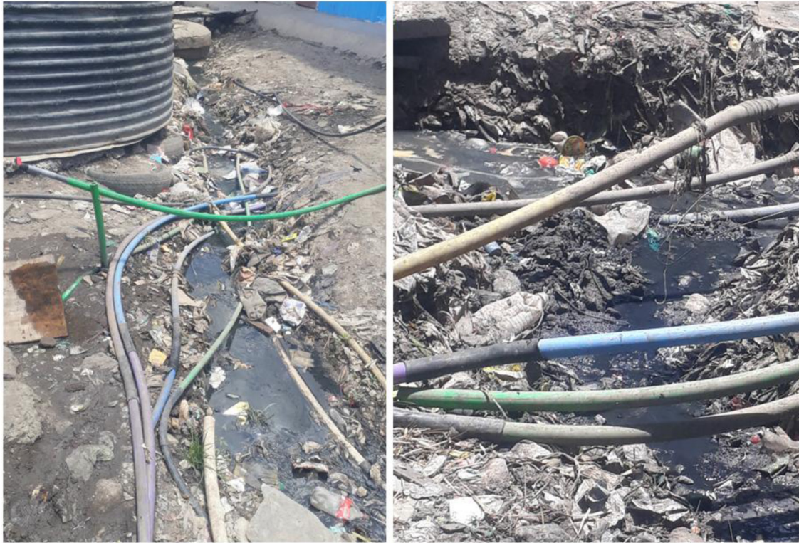
Fig. 3. Clean water pipes laid in an open sewage and highly polluted environment in Kibera informal housing. This image was taken in Kibera informal housings and shows refuse and raw sewage at the central communal water point. Clean water supply pipes are also laid in an open sewer and refuse, which pose a risk of contamination when there are leaks and through pipe joints. Therefore, there is a high possibility that the water supply in this informal settlement is already contaminated and is a source of microbial contaminants.
