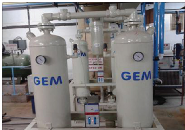
Figure 3: Installation of dryers, filters, electronically operated drains
