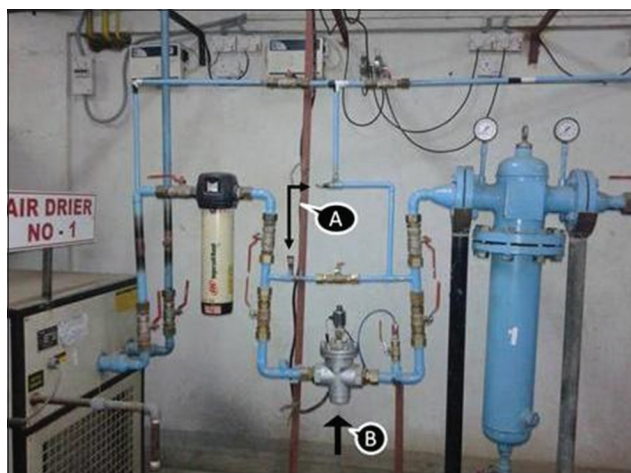
Figure 2: Air dryer bypass valve removed (A) and installation of air stopper valve assembly (B)
