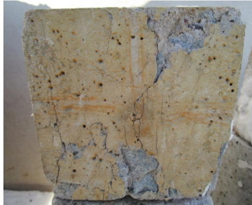
Figure 7. Sulfate corrosion for crumb rubber concrete.
