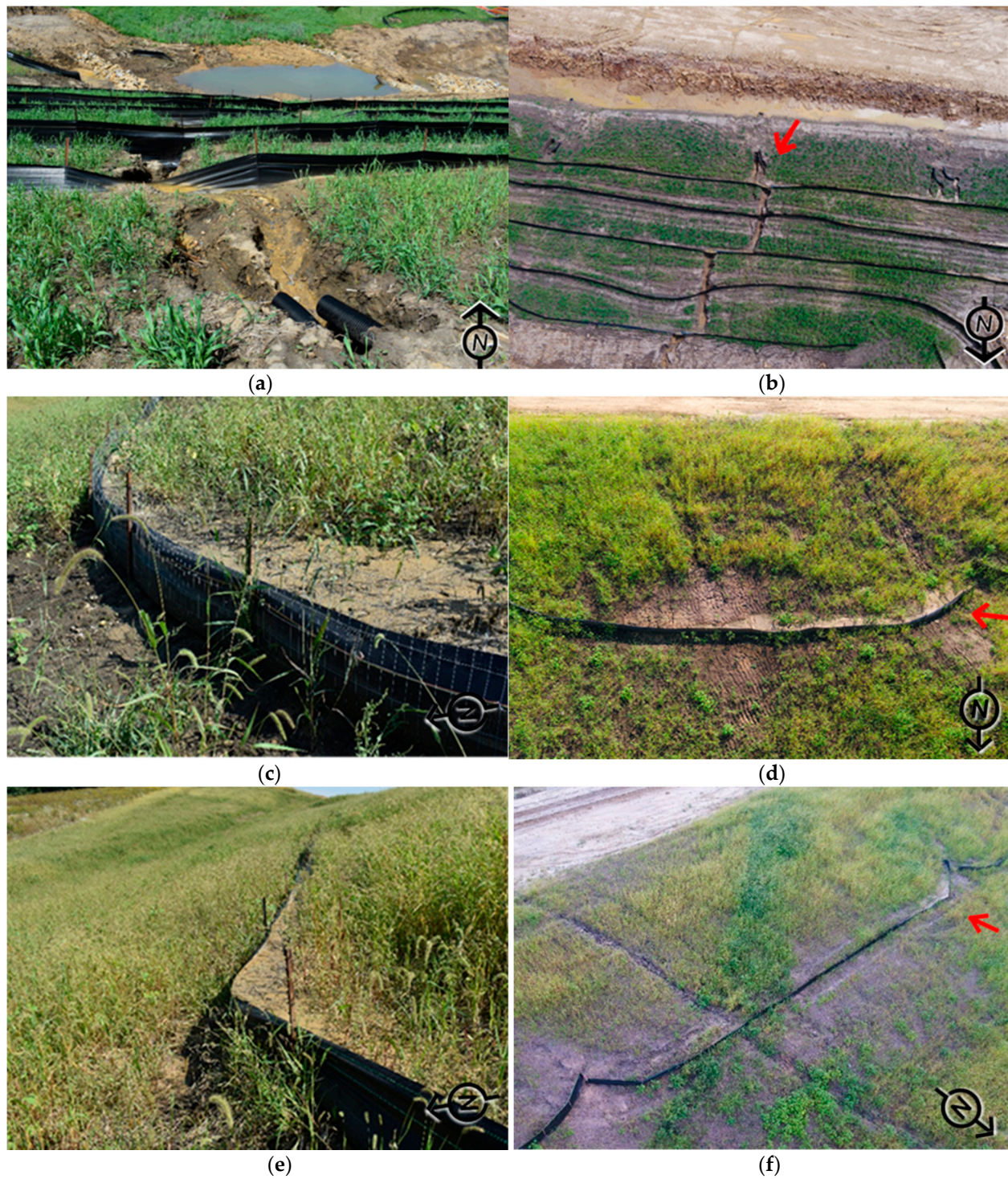
Figure 6. Comparison of silt fence inspection documentation: (a) overtopping failure (ground perspective); (b) overtopping failure (aerial perspective); (c) sediment accumulation (ground perspective); (d) sediment accumulation (aerial perspective); (e) sediment accumulation (ground perspective); (f) sediment accumulation (aerial perspective)
