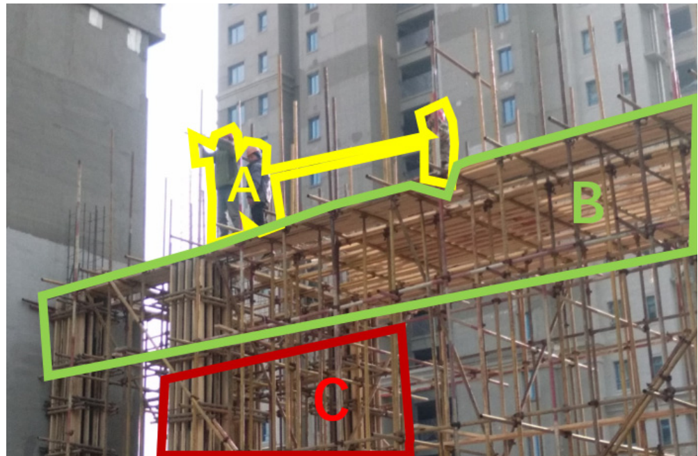
Figure 6. PPE failure (Hazard #3).
