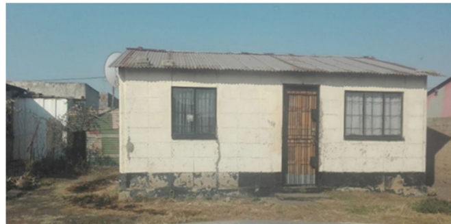
Figure 3. An archetypal Kathorus apartheid era- matchbox- house constructed in the early 1960s, housing between one to six occupants. The houses were typically 40 m 2 in area, and were constructed with low-grade clay brick. The houses either had corrugated or asbestos roofing, and four windows (two in the front and two at the back).
