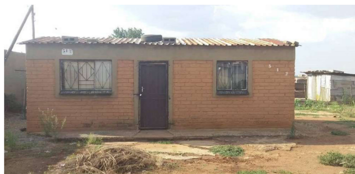
Figure 4. A distinctive RDP house in the Kathorus area, built in the mid-to-late 90s, housing between one to five occupants, with an area of about 36–40 m 2 . The houses were made with cement bricks. The house had asbestos roofs and three windows (at two windows front and one at the back).
