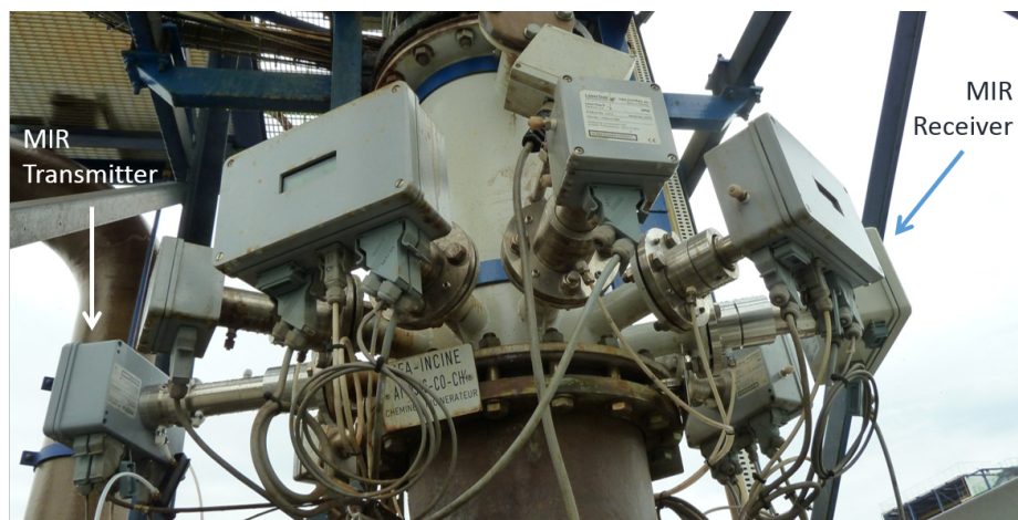
Figure 10. Installation of the mid-infrared NO sensor on a stack of an Arkema Forane-plant near Lyon (France). This photograph has previously been used in the presentation of Kaspersen et al. [17].
