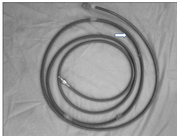
Figure 1: Nitrous oxide pipeline with arrow showing a dilated segment
