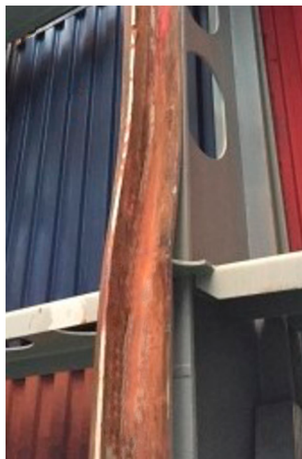
Figure 3. Example of a damaged vertical cell guide.
