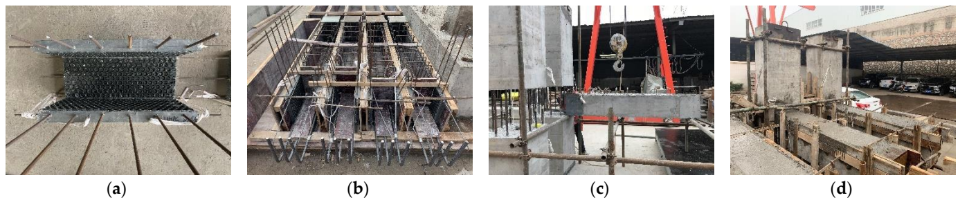
Figure 3. Manufacturing of the precast specimens. (a) Making UHPC shells, (b) fabricating beams, (c) installing beams, (d) pouring concrete.
