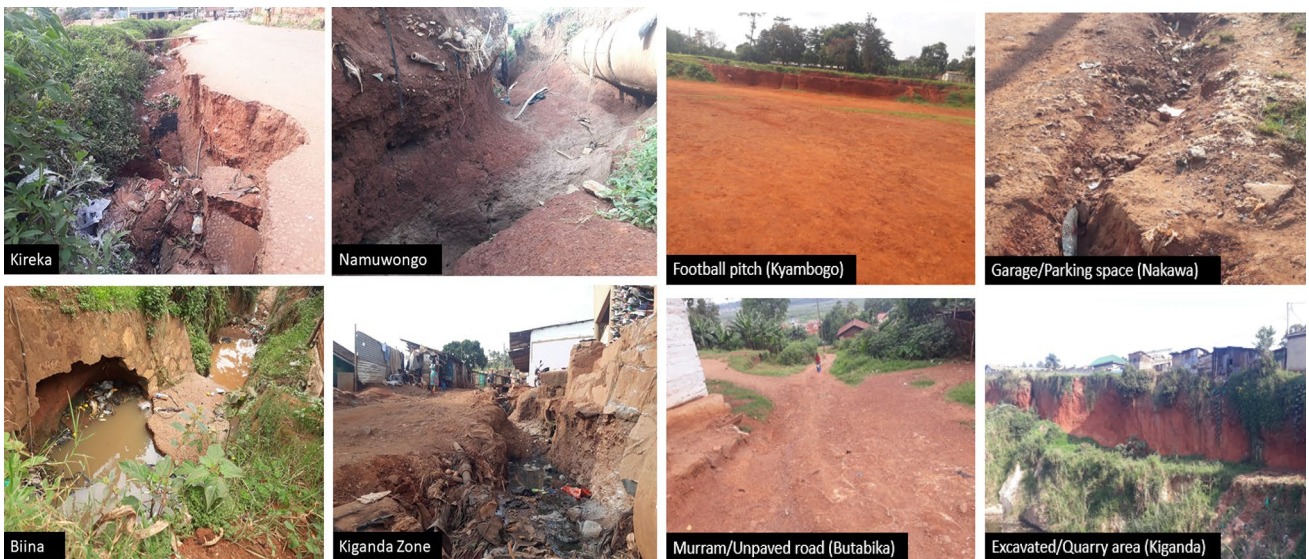
Fig. 12 Other identified erosion hot spots from field walks
