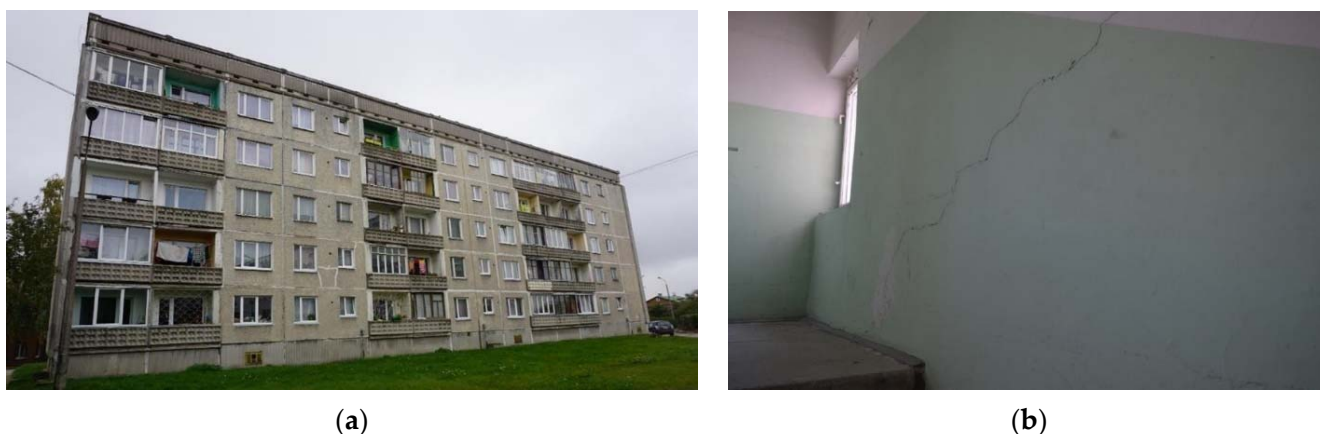
Figure 9. Cracks in residential buildings: (a) cracks in building façade panels; (b) cracks in building loadbearing walls.
