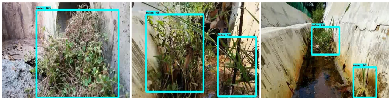
Figure 16. Bushes detection on real time drain inspection field test (day).
