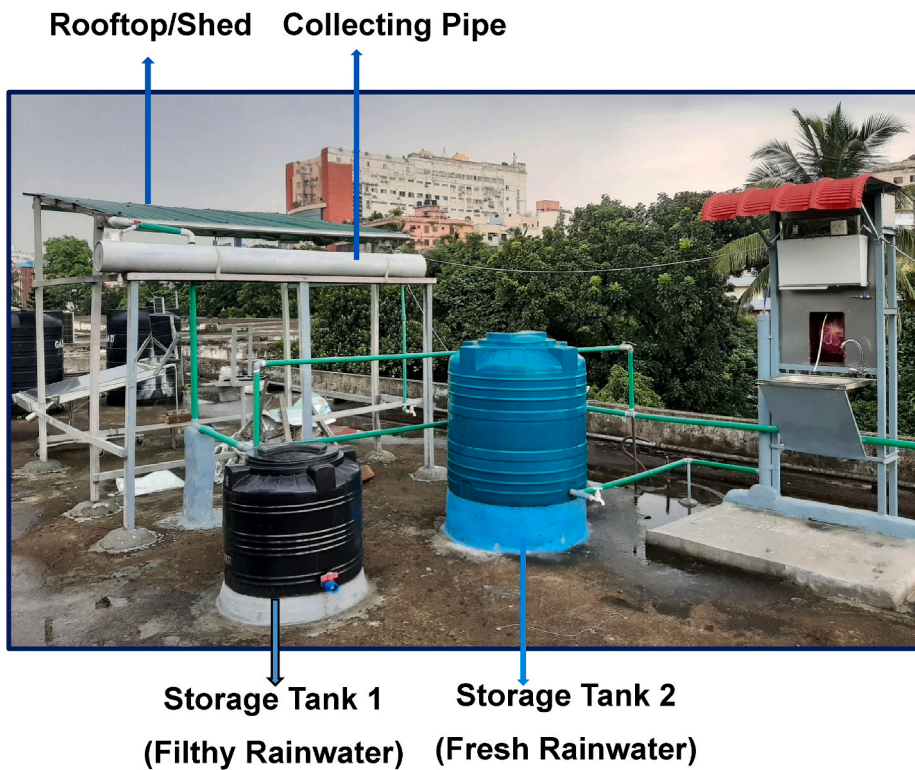
Fig. 3. Pictorial representation of the fabricated rainwater harvesting system on the rooftop of INARS, BCSIR, Dhaka, Bangladesh.
