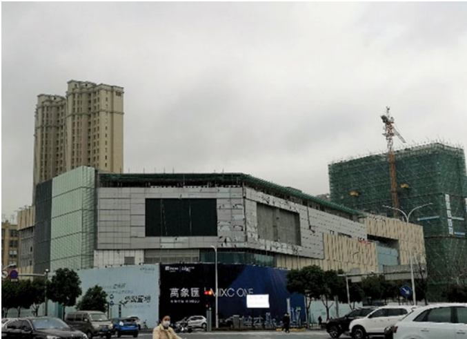
Fig. 5.22 The city's many constriction sites were on halt for an extended period due to multiple facts, partly associated to limited resources and workforces or the need for larger mobility of workforces from other parts of the province and other provinces. Source Ali Cheshmehzangi
