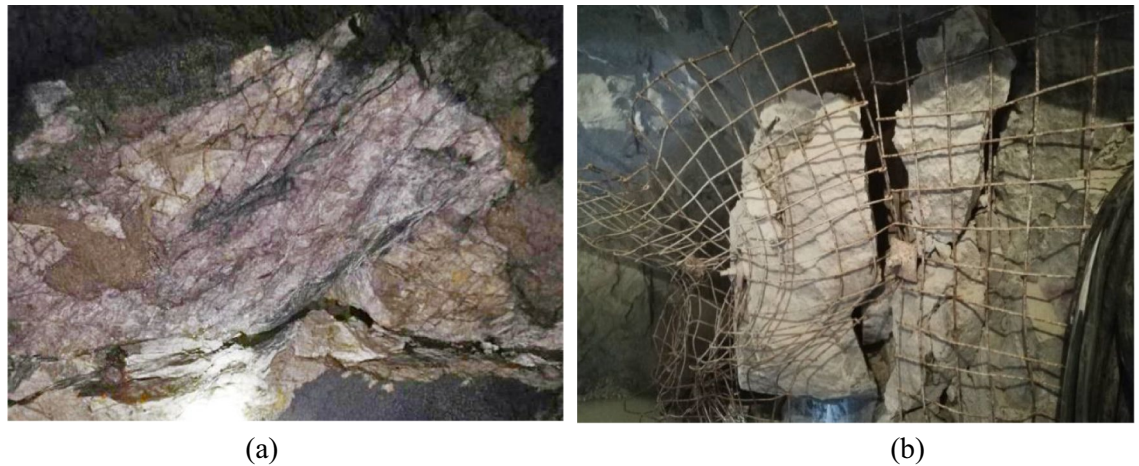
Figure 12. Failure characteristics of roadway surrounding rock in Xincheng Gold Mine. (a) Plate cracking of surrounding rock in roadway side, (b) the falling off of the surrounding rock after plate cracking.
