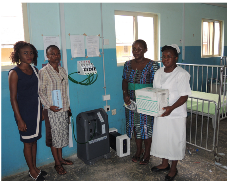
Technician, doctor, and nurse in Ondo state, Nigeria, with new oxygen installation including oxygen concentrator with power stabilizer, oximeter, flowmeter stand, distribution tubing, oxygen analyzer, and user guides. © 2016 Oxygen for Life Initiative
