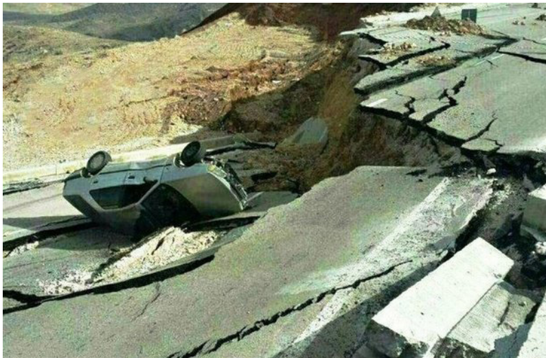
Figure 1: Land subsidence in a road, Fars province, southern Iran
