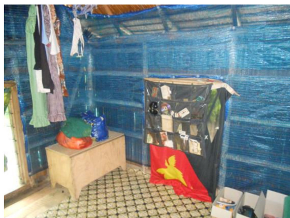
Figure 6 The interior wall of an Islands village house four-weeks post ZeroVector® ITPS installation.
