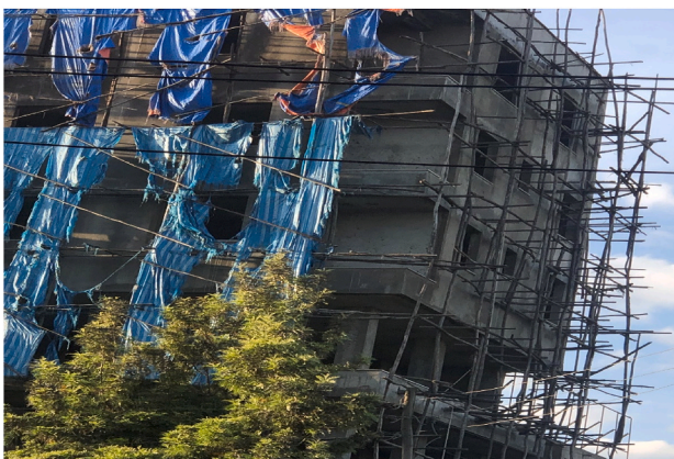
Fig. 2. Building under construction in Ethiopia showing weak wooden scaffoldings.
