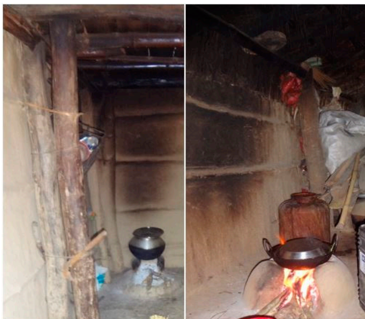
Figure 2. Picture showing black layers of smoke on the kitchen wall and ceiling.
