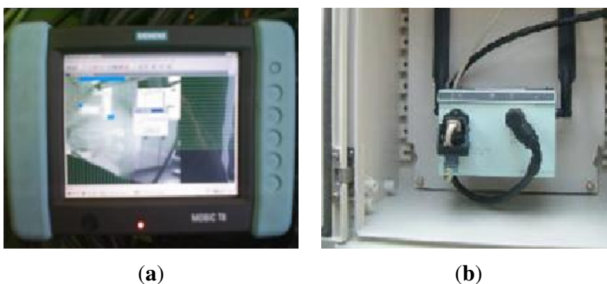
Figure 22. Remote wireless console to work outside of the cabin. (a) Panel that offers the same functions that the graphic interface installed inside the protection cabin. (b) The access point that is connected to the Control Unit and located at the cabinets of the primary structure to which the wireless console of the operator is remotely connected.
