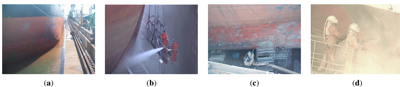
Figure 2. The maintenance works of a ship hull. (a) Beaching; (b) Ship Hull Desalination; (c) and (d) Grit-blasting cleaning process.
