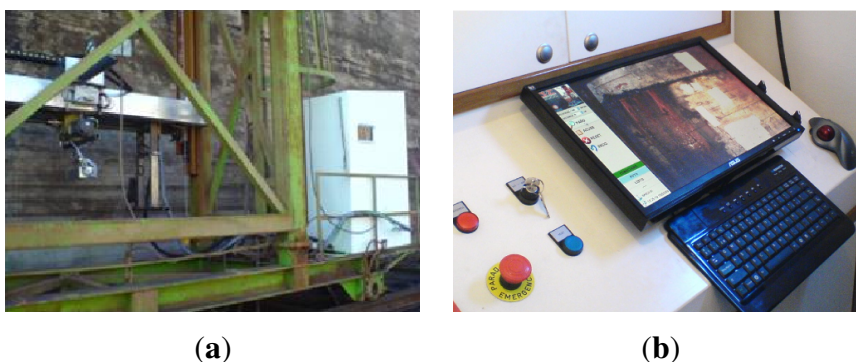
Figure 21. (a) Assembly of the system on the dry dock and view of the control cabin; (b) Detailed image of the Supervision Unit graphic interface installed inside the cabin.
