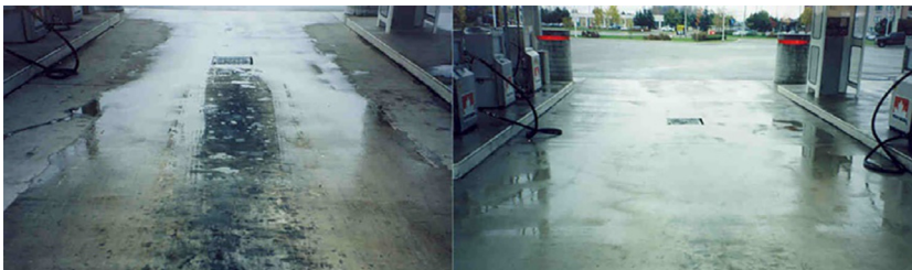
FIGURE 15.4 Photos of a truck fueling bay before (left) and after (right) microbial cleaning [39]. (Courtesy Worldware Enterprises, Ontario, Canada).
