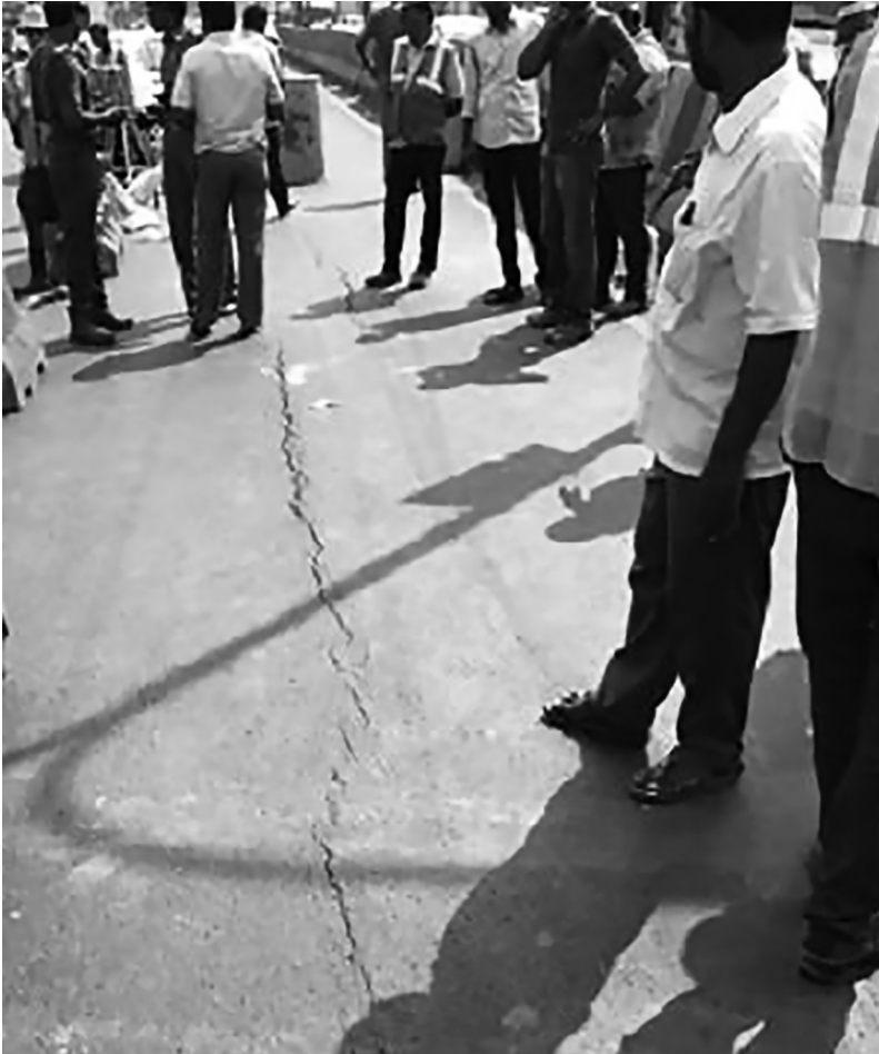
FIGURE 2 Cracks in Anna Salai, April 2017 (The News Minute 2017).
