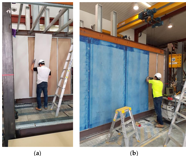
Figure 5. (a) Representative interior wall with gypsum plasterboards on both sides of the studs, (b) exterior wall with gypsum-board on inner side and cement-board at outer side.
