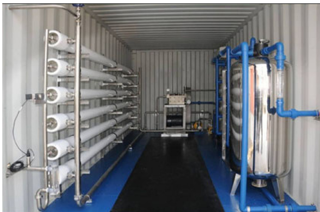
Figure 5. Internal view of a containerized seawater RO desalination unit.
